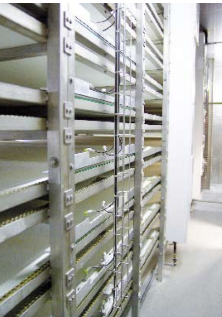
The exactly air-conditioned multi-deck belt proofer has own loaders and unloaders.
